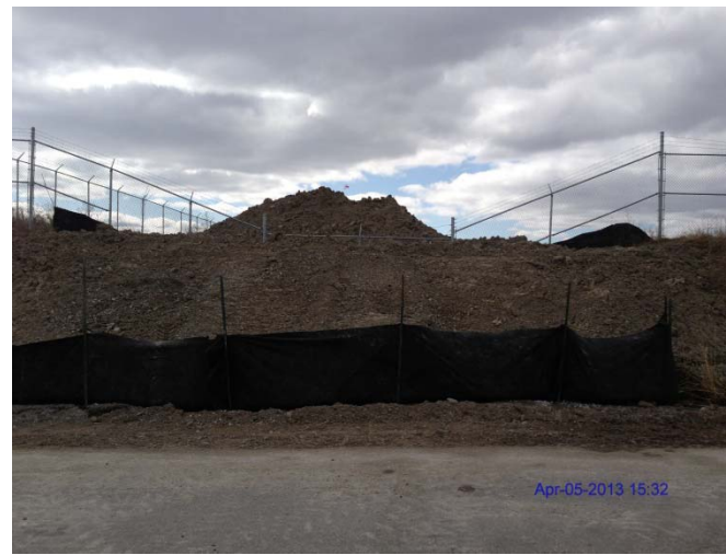
Photo 16: Looking west at east side of perimeter fencing at the southeast corner showing silt curtain installed
