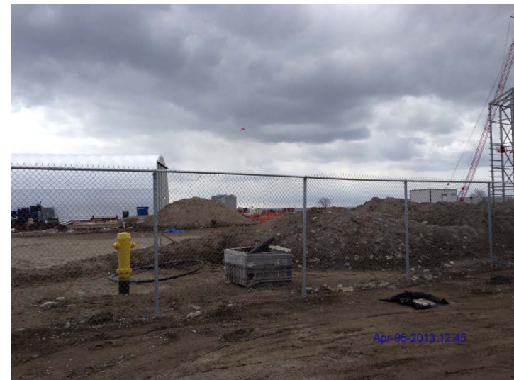
Photo 6: Looking south (showing temporary soil stock piles from parking area) and catch-basin with silt curtain protection
