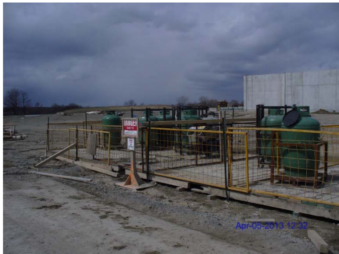
Photo 13: Looking northwest showing compressed gas storage
