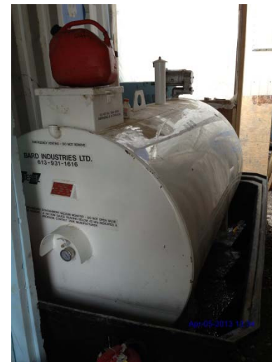
Photo 26: Liquid fuels tank with secondary containment
