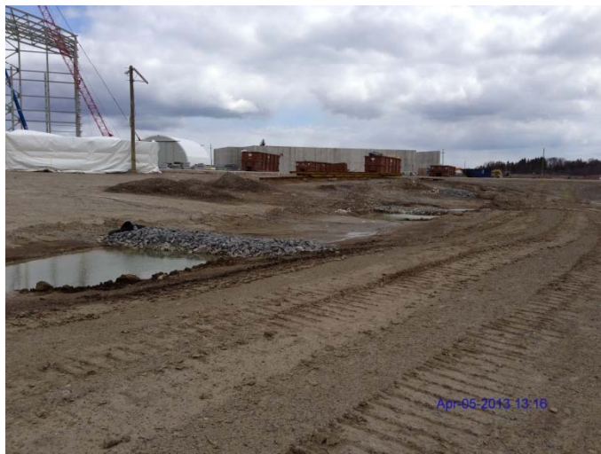
Photo 19: Looking east showing erosion control and sedimentation measures in west drainage ditch
