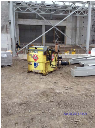
Photo 23: Fuel dispensing equipment north of building.
