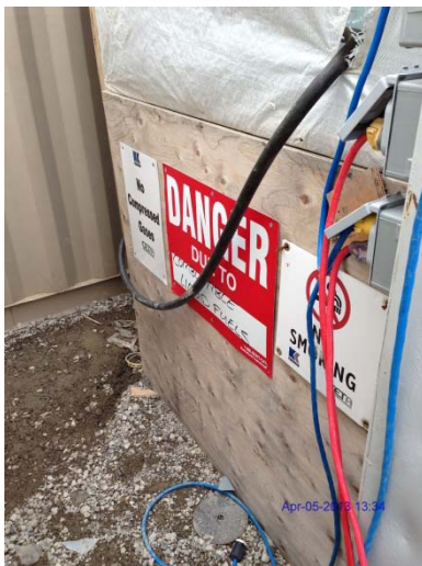
Photo 25: Signage on liquid fuels enclosure identifying no compressed gas storage
