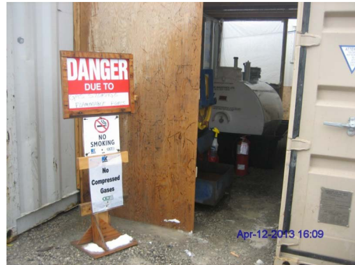
Photo 28: Liquid fuels storage area showing removed compressed fuel tank as reported by Region of Durham staff on 13/04/12
