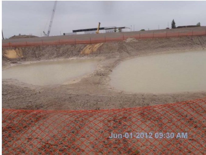
Photo 24: Looking east across west storm water management pond, showing erosion control features.
