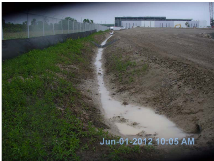
Photo 30: View of north fence line and drainage swale looking east. Rock check dams and culvert crossing under temporary road access to the west.
