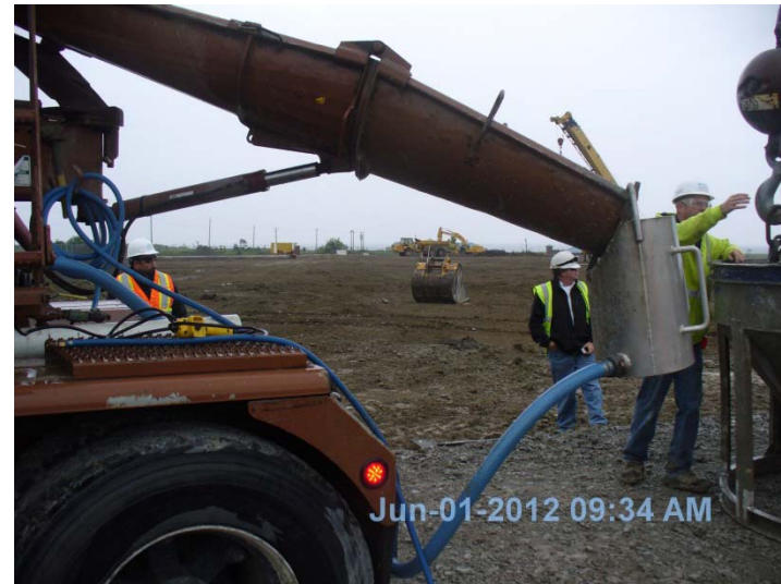
Photo 33: Recirculating water bucket and pump to capture wash water from cement trucks, no on-site discharge.
