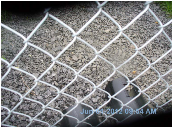
Photo 19: Temporary discharge gallery from west storage pond immediately outside of south fence line near southwest corner.
