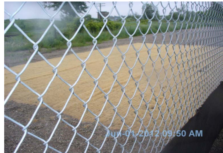
Photo 12: Erosion and sediment control mat outside of fence; wildlife corridor beyond worked ground.
