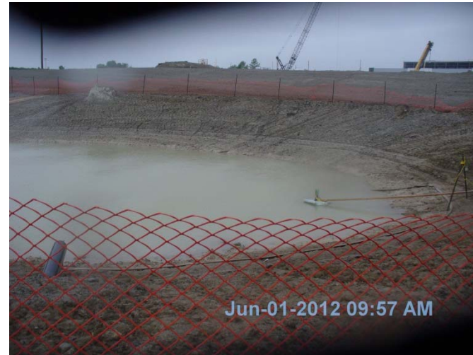
Photo 25: West storm water management pond showing discharge pipe in left foreground and temporary pump to maintain a low water level in the pond.
