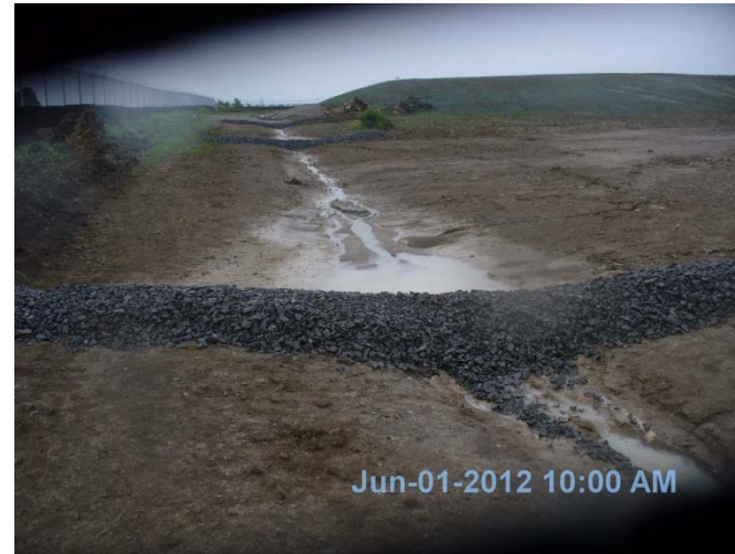
Photo 22: Rock check dams along drainage swale flowing south adjacent to the west fence line.
