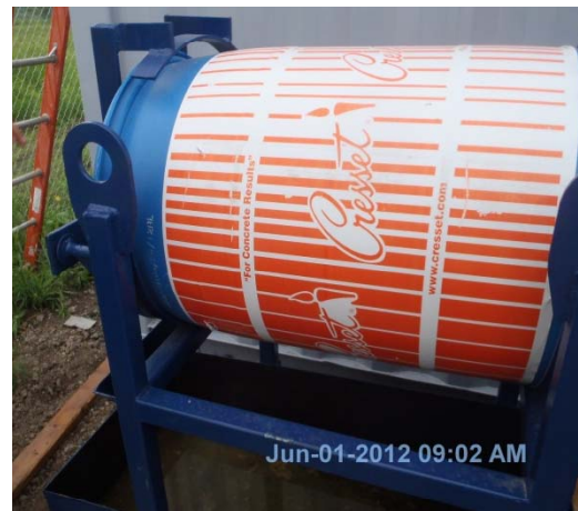
Photo 35: liquid material handling with secondary containment.
