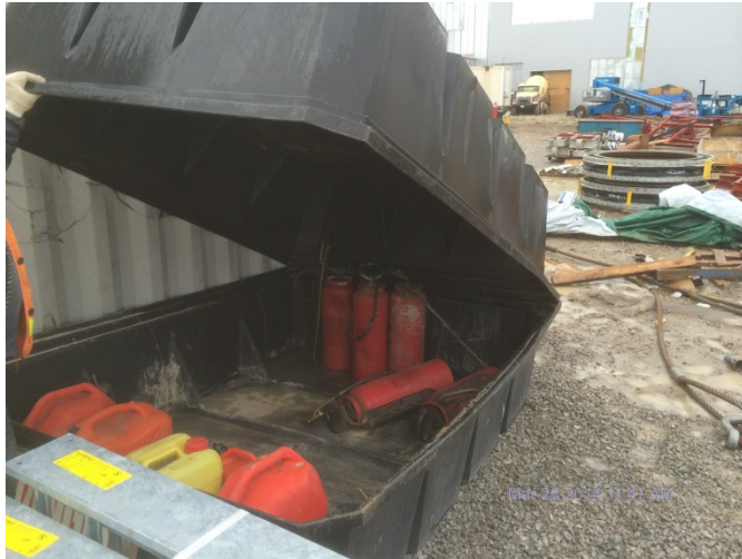
Photo 15: Liquid fuel storage west of main building.
