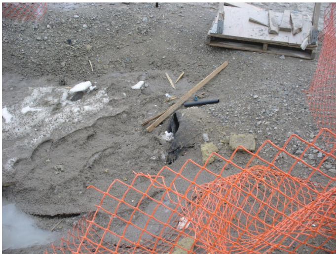
Photo 27: Drainage ditch south of visitors centre with debris.
