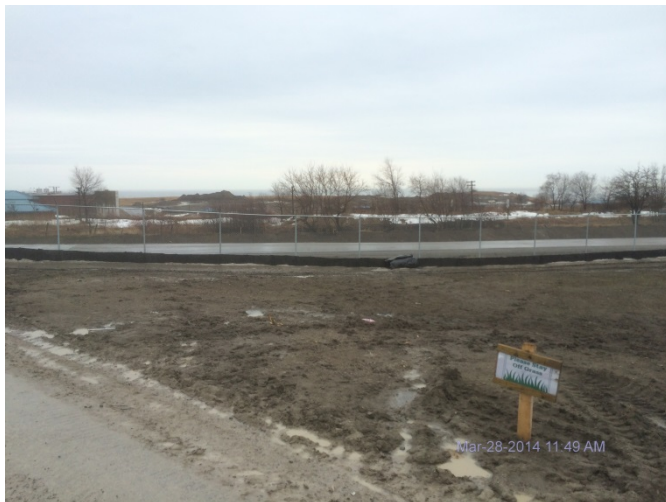
Photo 17: Looking south, across the south portion of the site, showing hydro-seeded graded areas.
