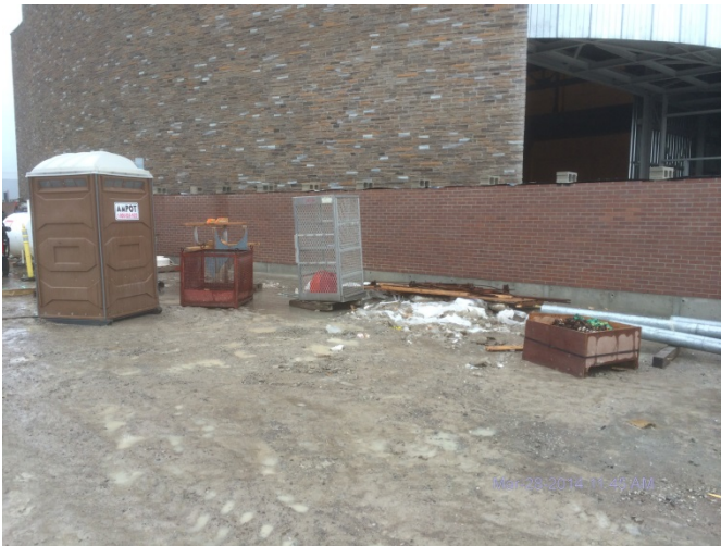
Photo 12: Liquid fuel storage north of main building.
