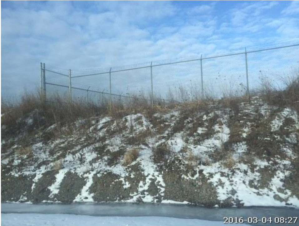
Photo # 03 looking west from Osborne Road at southeast corner showing closed access
