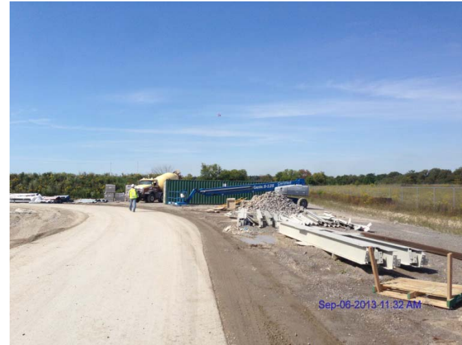
Photo 10: Looking west along the north of the site showing paved road, construction materials and equipment
