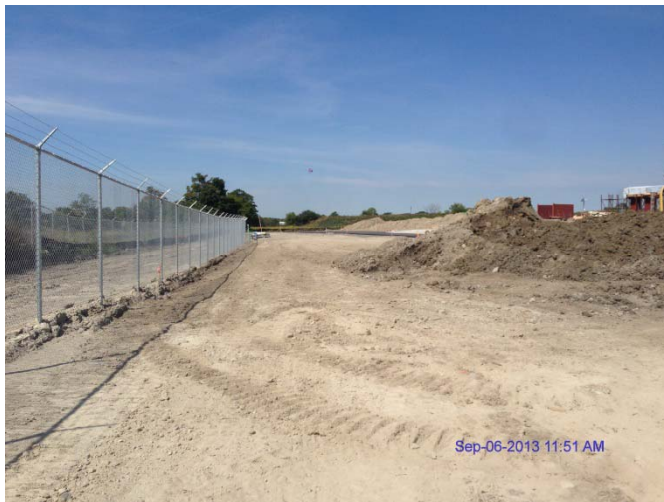
Photo 19: Looking west along south property line showing original fence, re-aligned fence and temporarily stockpiled soils
