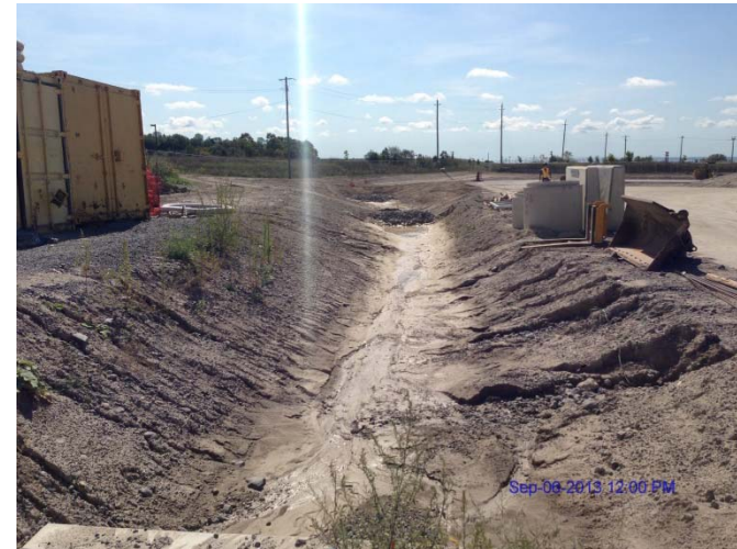
Photo 22: Looking southeast along the property interior showing drainage ditch with rock check dam
