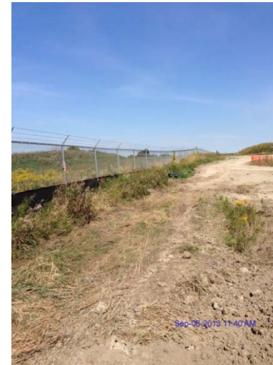
Photo 14: View north along west property line showing fence and silt curtain condition
