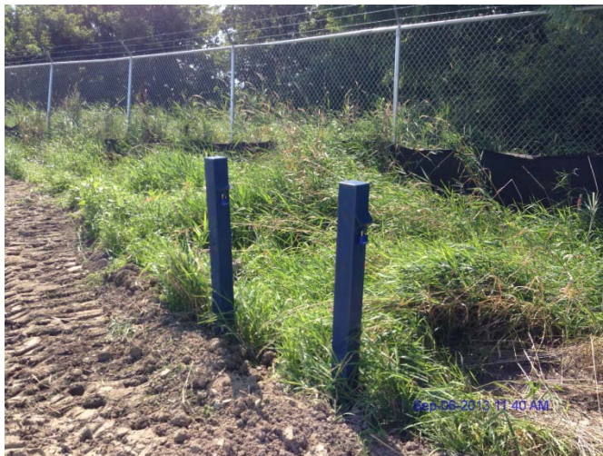
Photo 15: View of monitoring well condition in southwest corner
