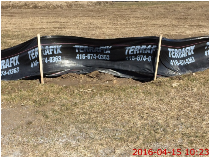
Photo 33: silt fence enclosing temporary sediment storage – in need of repair.
