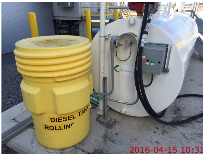
Photo 19: refuelling area with spill containment drum.
