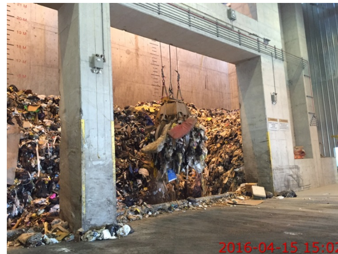
Photo 20: waste tipping building of gantry crane loading waste into receiving hopper.
