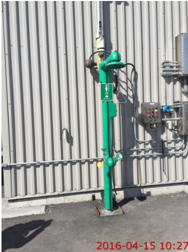
Photo 17: emergency wash station next to lime loading station.
