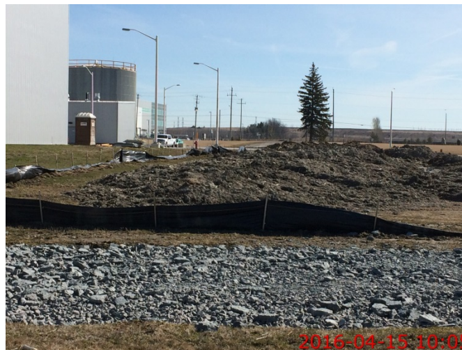
Photo 32: storm water management pond sediments temporarily stored on site – silt fence enclosure in need of repair.
